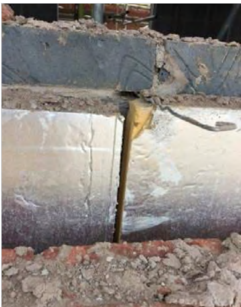
Examples of poorly installed insulation
