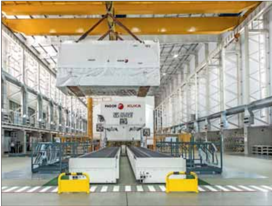
The press bed, weighing 120 tons, was lifted eight metres over the existing press line.
