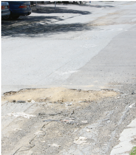
One of the many potholes that has been covered with sand.
