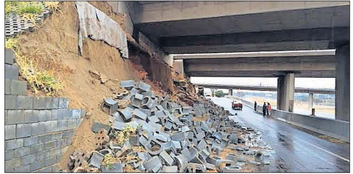
Heavy rain caused the hill to partially collapse next to the bridge on the N14/R55 to Krugersdorp on Saturday.
