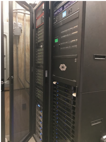
Racks in the main distribution frame (MDF) house more than 50 key AV/IT components in a very small space.
