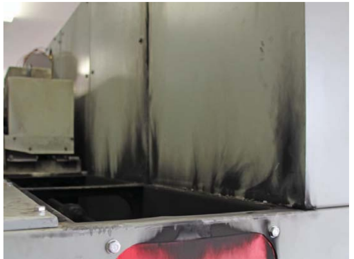
A busbar that burned out left many residents in the dark. Some of the damage is visible.
