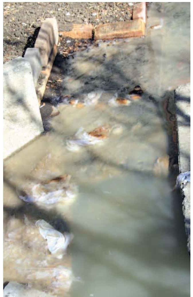
Human faeces flows from a manhole in a Secunda resident's yard.
